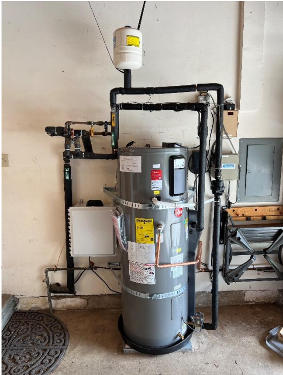
FIGURE 36. PHOTO SHOWING INSTALLED HPWH WITH MONITORING BOX
